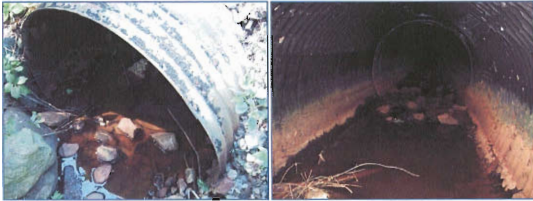
Photos 10 & 11: 48" Corrugated Metal Pipe inlet at Leitha Drive Swale Terminus C&C September 2010
