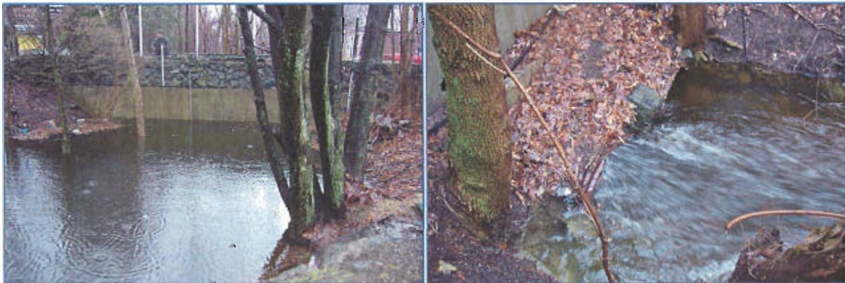
Photo 7 (Left): Upstream of Stearns Hill Road after rain event, C&C March 2010
